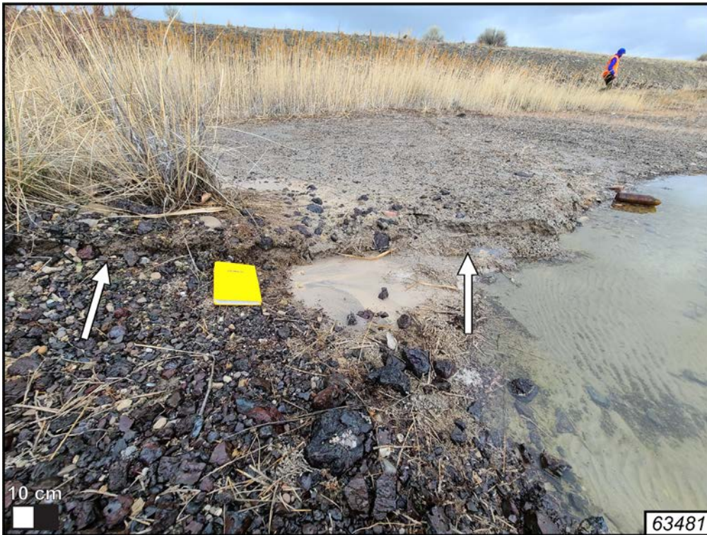
Figure 6. Subaerial sand boil (center of photo) and extensional ground crack with 2–3 cm of vertical separation (indicated by arrows) near the I-80/SR-202 interchange and Great Saltair event venue. Field notebook (10 cm wide) for scale. Resource ID from the Magna earthquake online clearinghouse labeled in bottom right corner of photo.
