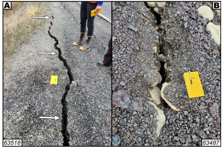
Figure 10. (A) Multiple cracks (shown by arrows) in the roadway base material along the Great Salt Lake State Park Marina Access Road. Primary crack shows approximately 3–4 cm of vertical separation. Field notebook (10 cm wide) for scale. (B) Close-up view showing approximately 30-cm-deep crack. Resource ID from the Magna earthquake online clearinghouse labeled in bottom right corner of photos.
