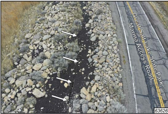
Figure 9. sUAS image of the Great Salt Lake State Park Marina Access Road showing an approximately 6-meter-long crack in the roadway base material (shown by arrows). Resource ID from the Magna earthquake online clearinghouse labeled in bottom right corner of photo.
