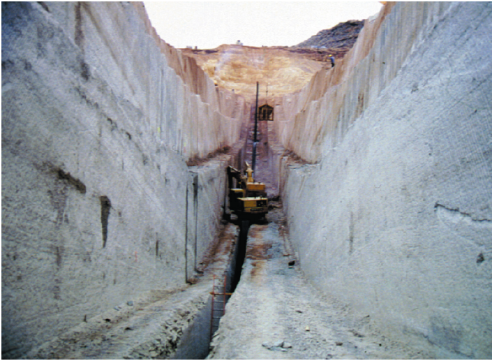
Figure 10. Cutoff trench being excavated at the bottom of the new Quail Creek south dam in January 1990. View east. Note seepage of water on left-side of trench. Photo by Bill Lund, Utah Geological Survey (retired).
