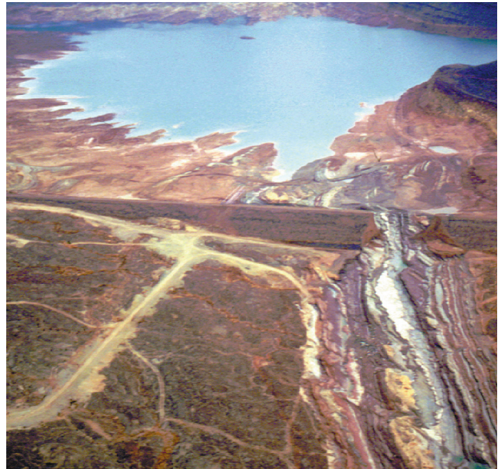
Figure 9. Quail Creek south dike, shortly after its catastrophic failure on January 1, 1989. Note how floodwaters scoured the bedrock clean of loose, overlying sediments just below the dike. Photo by Ben Everitt, Utah Division of Water Resources (retired).
